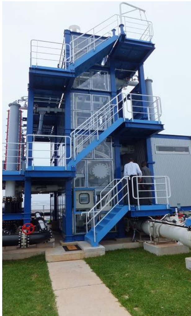
Figure 1: THE BEAUTIFUL POTENTIAL OF “DOMINIQUE”: A magnificent 100 KW Ocean Thermal Energy Conversion Pilot Plant located on Kumejima Island, Japan
